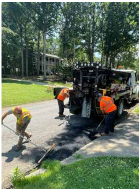
The Public Works Streets & Sewer Division maintains 85 miles of city-owned streets, 113 miles of sewer and more than 4,000 manholes.
